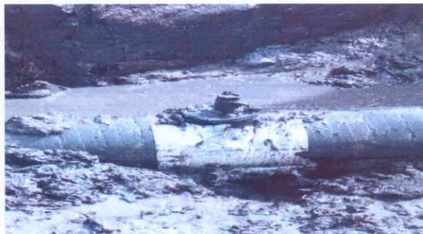
SPILL POINT AFTER EXCAVATION
